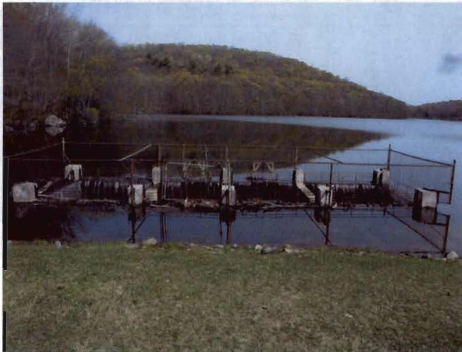
Figure 2-3: Seven Hills Dam - Drop Inlet Spillway
